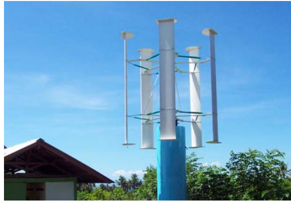
The 3 kW vertical axle windmill. This type of windmill is not affected by turbulence. The energy is used to power the center
