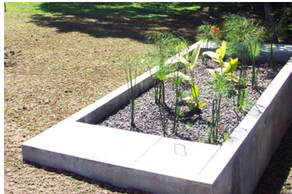
The wastewater garden that transforms the grey water from the biodigester to clear water that is nearly bacteria free and feeds a fishpond
