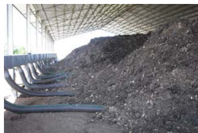
Aeration ducting. Volume control with butterfly vales at each inlet
