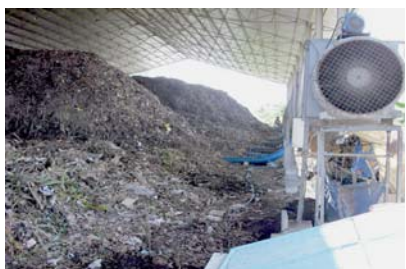
Forced aeration with blower
