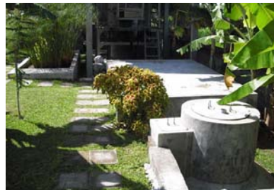
Biogas reactor for facility toilets used for cooking
