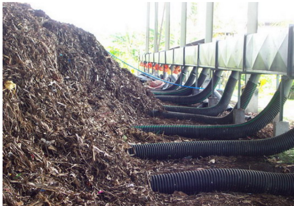
Industrial Scale Composting: Blowers assure an aerobic process that reduces greenhouse gasses
